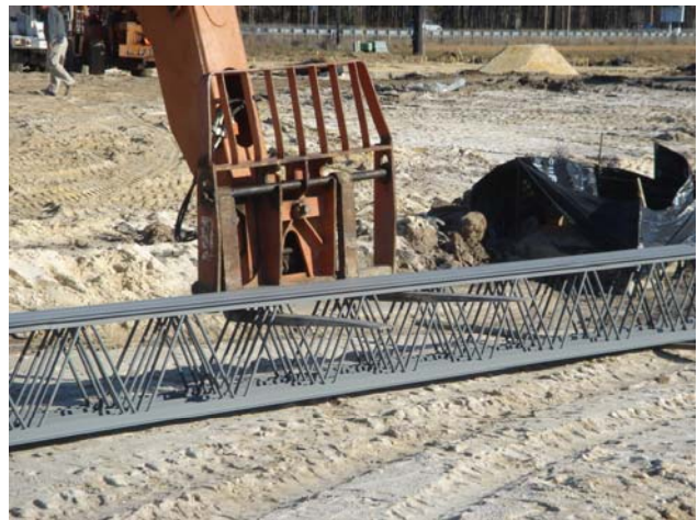
Figure 8 Improper joist handling – Fork on left is wedged between two web members, could damage webs
