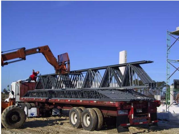
Figure 5 Unloading a bundle of Joist Girders with a fork-type lift typically available on construction sites
