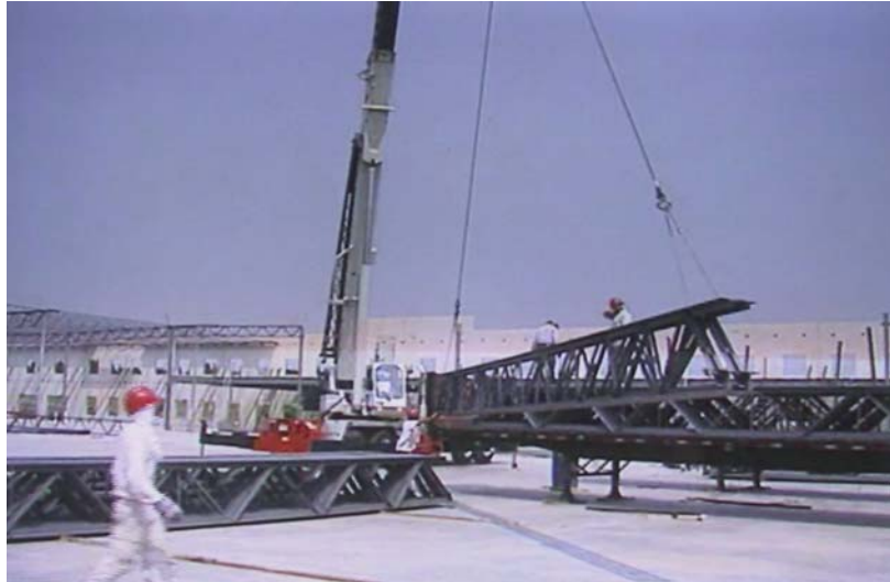
Figure 4 Lifting with a crane using two chokers configured in a basket hitch and two-way spreaders
