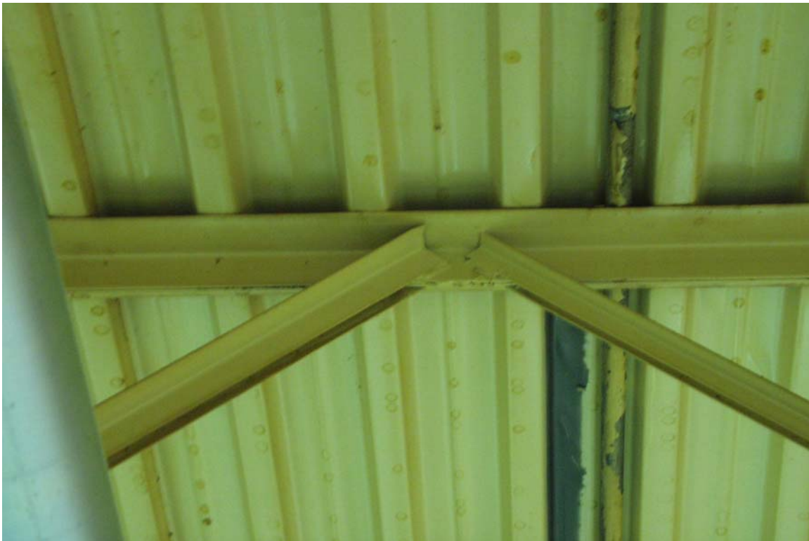
Fig. 5 Angles interfering with Top Chord Reinforcement
