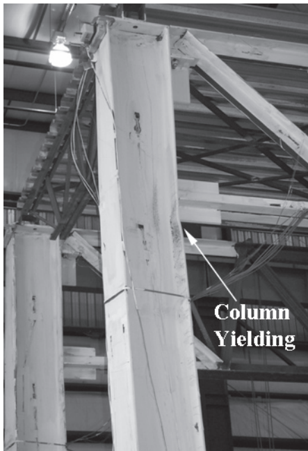
Fig. 11. Plastic hinge formation at the column.
