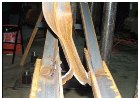
Figure 12 Fracture of Web Member at Bottom Chord Connection
