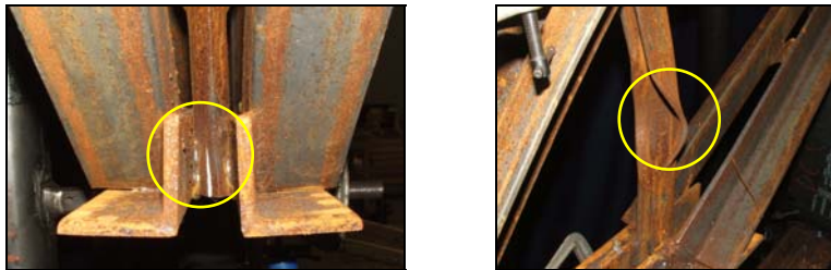
Figure 2 Buckling of crimp transition zone and member fracture (J2200-R1)
