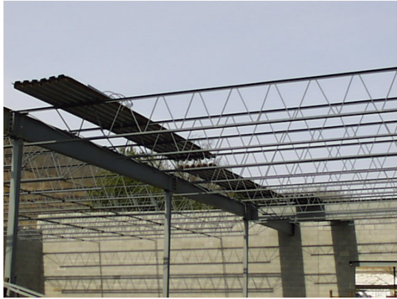
FIGURE 1 CONSTRUCTION LOADS SET ON UNBRIDGED, UNANCHORED JOISTS
